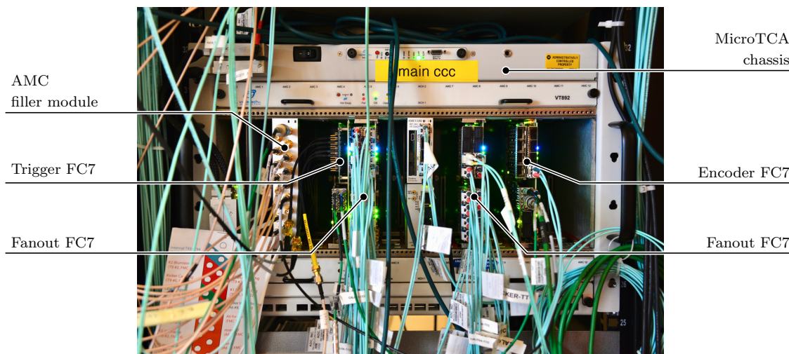
Figure 3.4: The Clock and Commands Center (CCC), implemented in a MicroTCA chassis with four FC7s. The multi-mode, optical fibers in teal from the two Fanout FC7s are routed through two patch panels to the calorimeter stations and some of the auxiliary detector systems. Note that, in place of the HiTech Global SMA/LVDS FMC, the Trigger FC7 shown is outfitted with an FMC custom-designed by Cornell University, which was used after Run 1.
